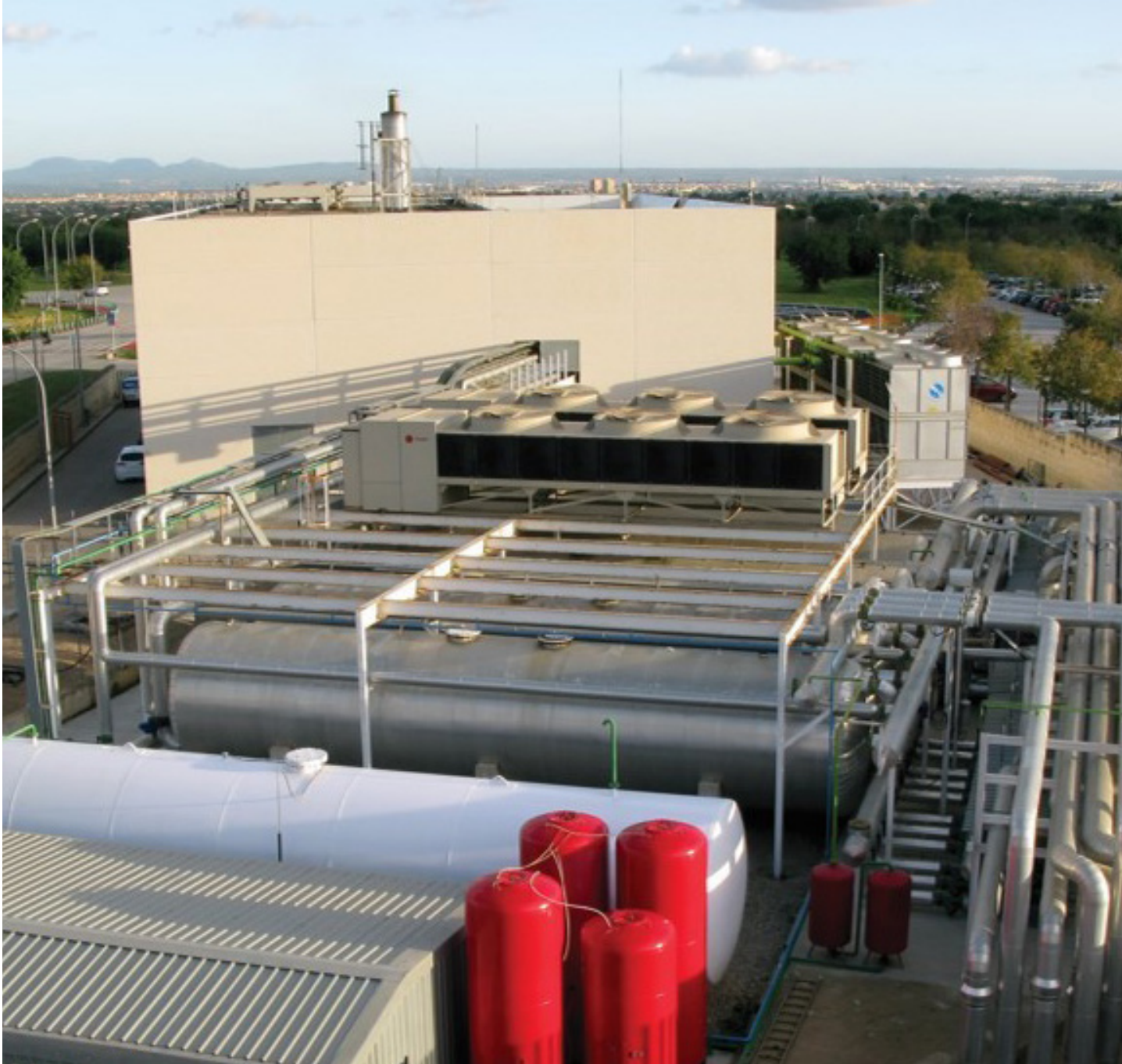
Parc Bit has an advanced tri-generation plant that supplies the area with heating, cooling and electricity.
